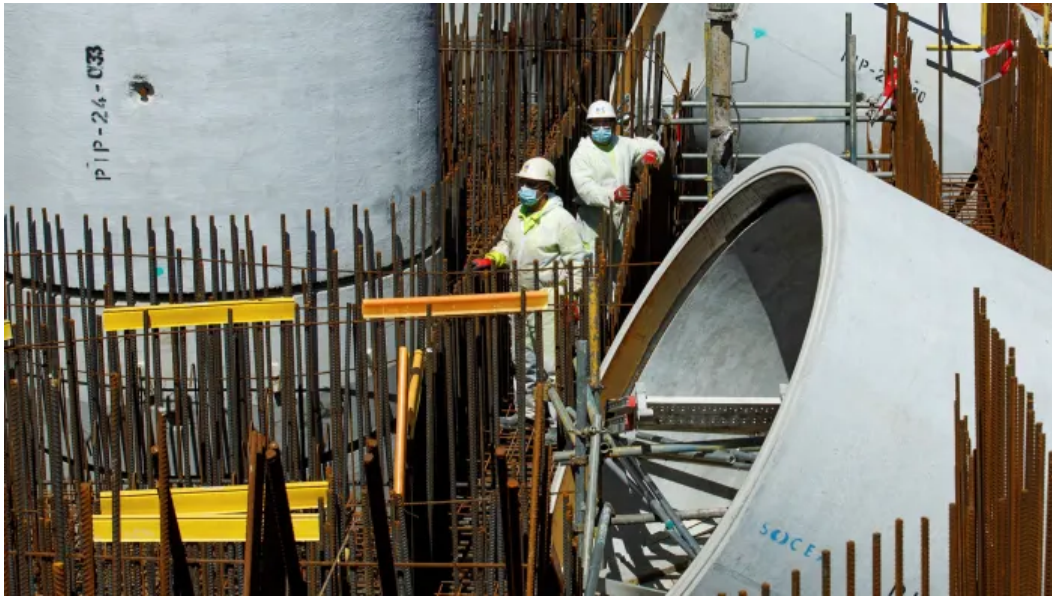
Contractors work on construction of Hinkley Point nuclear power station in Somerset. The two giant French-designed plants have a rating of 1,630MW each © Bloomberg
